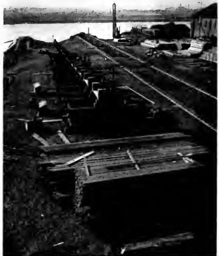
Laying out berths for new construction at the Pusey and Jones plant, Wilmington, Delaware.
